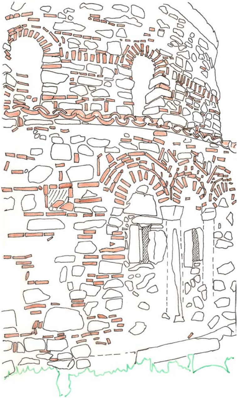
Fig. 55. Paravola, Panagia church. Drawing of a section of masonry in the apse viewed from SE.
